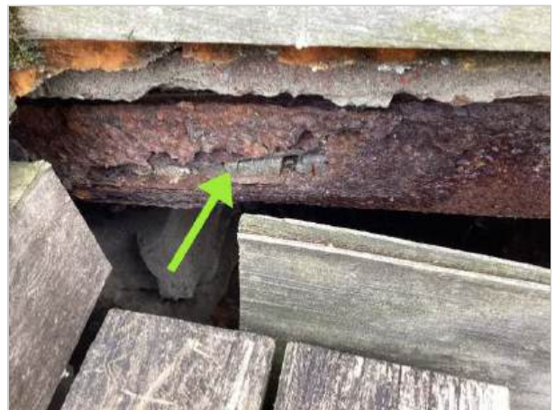
Rusted horizontal support
