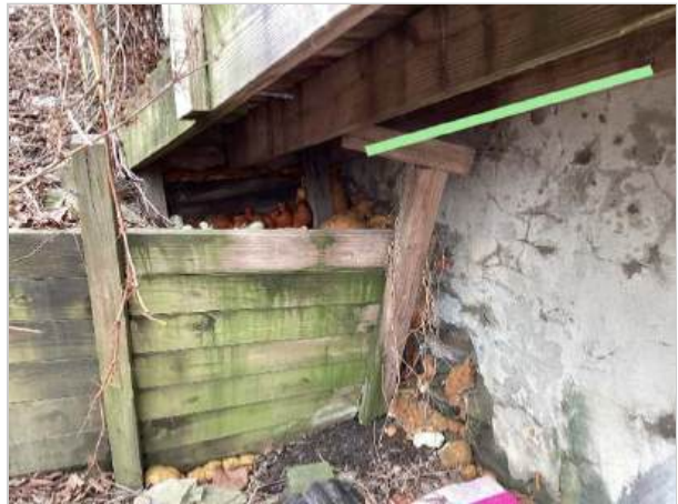
No evidence of bolts on front of ledger
