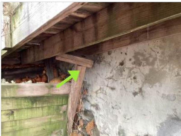
Loose support post
