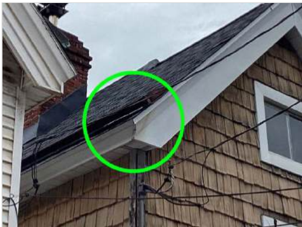
Evidence of leak
