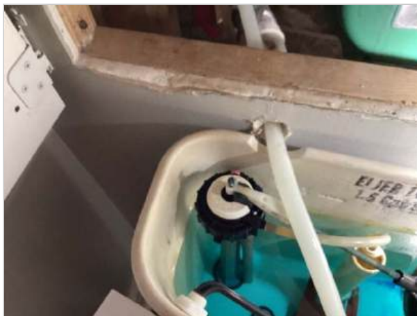
Drains to toilet tank
